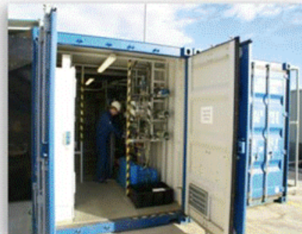
Oil Field containerized unit (UF + NF)
