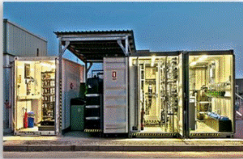
Water Reuse Platform (UF + RO)
