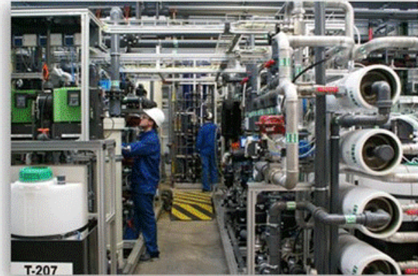
Industrial Water Platform (UF + RO + IER)
